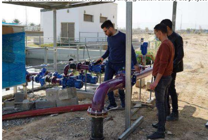
Fig.16 The pumping station set up by MEDISS at the WWTP of Jericho
