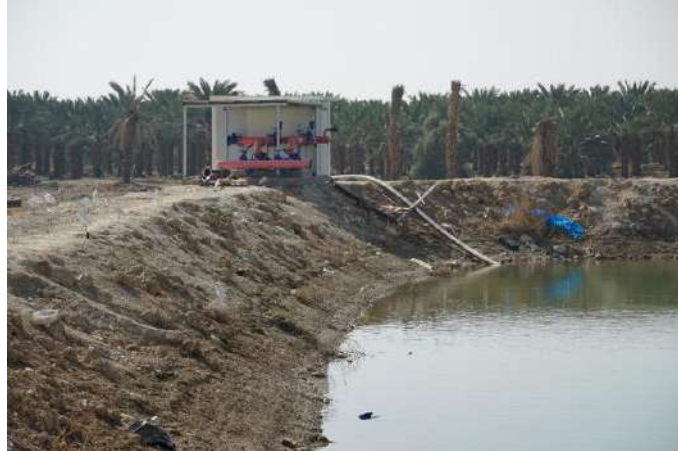
Fig.15 The MEDISS reservoir: detail of the pumping station built by the project
