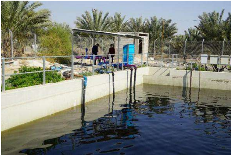
Fig. 10 The "irrigation tank" at the WWTP of Jericho. Pipelines and pumps of the single farmers who buy this water are shown. The pipeline of the MEDISS project is visible as well, under the roof
